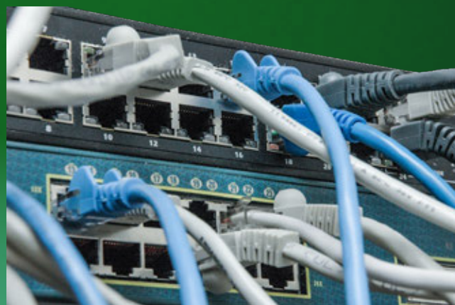
Ethernet cables plugged in to Ethernet switches in a server room. Photo by Jon 'ShakataGaNai' Davis, Wikimedia Commons
